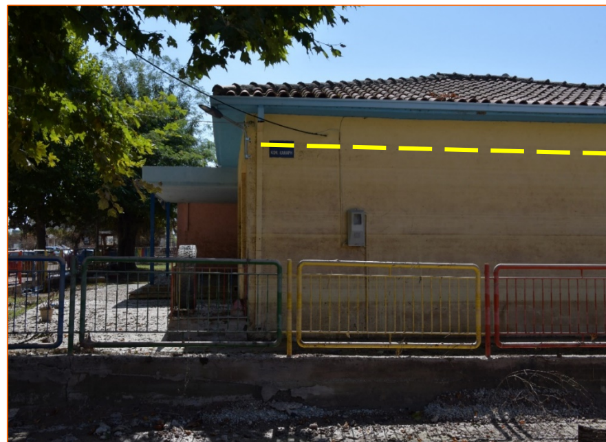
The water level (yellow mark) from the flooding has been imprinted on both the exterior and interior walls of the school.
